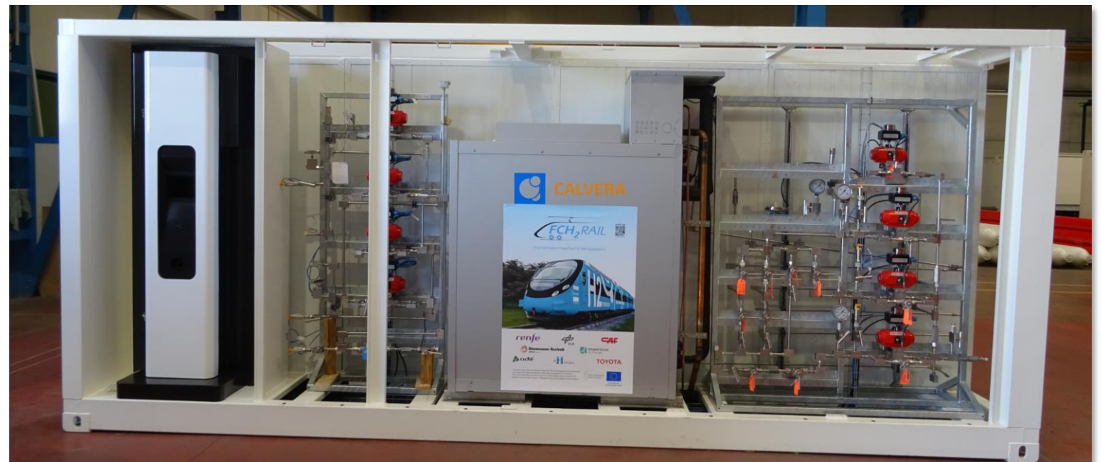
Container with dispenser, pressure control and control system for the HRS
